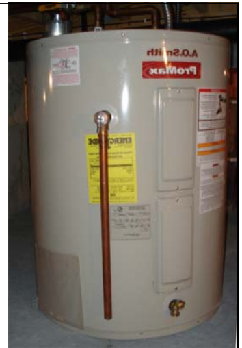
Electric Water Heater
