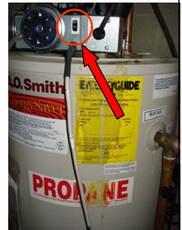
Power Vent Gas Water Heater
